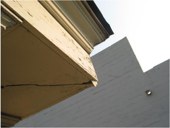
Fascia at corner. Paint flaking, but board appears to be solid.
