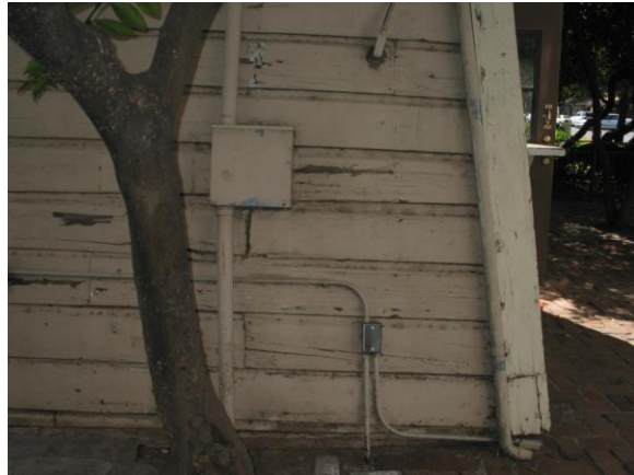
Cracked siding, electrical boxes, corner trim
