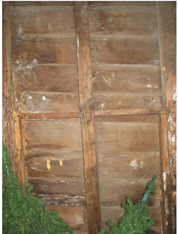
Inside studs, rotted, and in some places can see through siding joints. Note the 2X4's scabbed to inside of 4X4 studs that are now rotting too.
