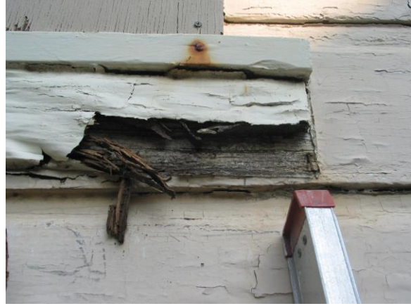
Rotted trim board at window
