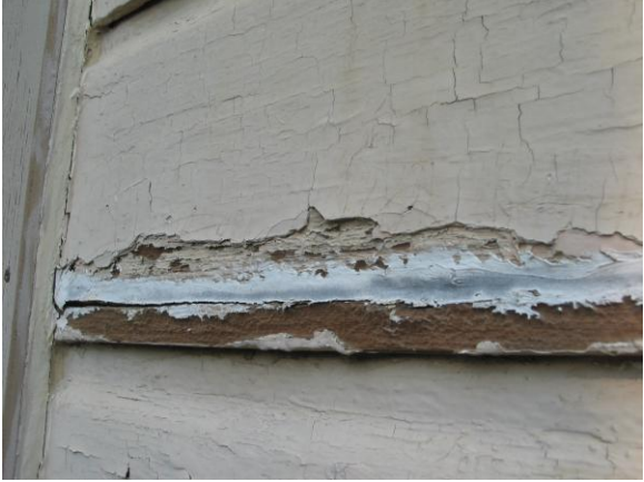
Siding, showing wood deterioration and crack
