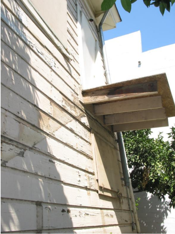
Old balcony added at second level Stairway removed Siding rotted
