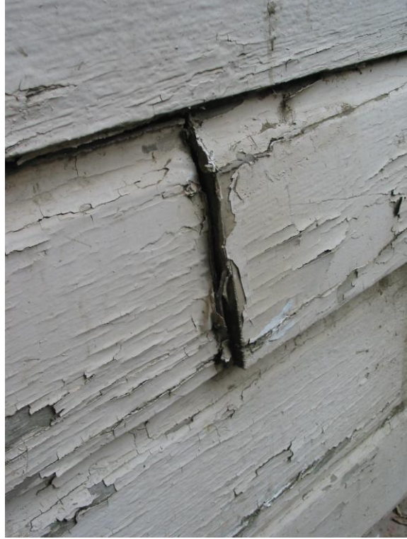
Siding, showing board pulling loose from rot
