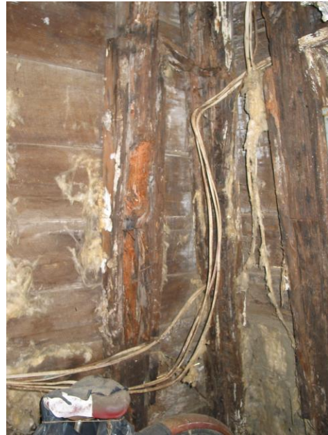
Dyrotted interior studs
