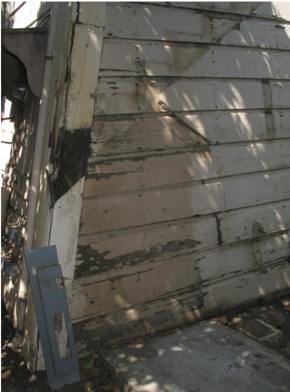
Rotted siding behind trim
