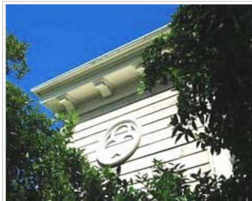
The Tank House - Upper Decorations & cornice under the tank deck. See also the Tank House
