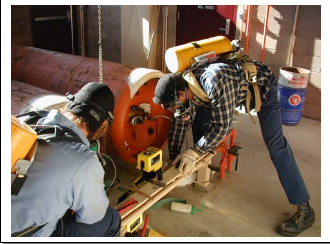
Sulfur dioxide tank exchange at the WWTP.
