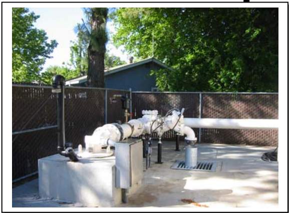
City Water Well located at 1812 Manzanita Lane.
