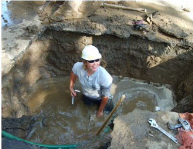
Service Line Break - Hawthorne Dr.
