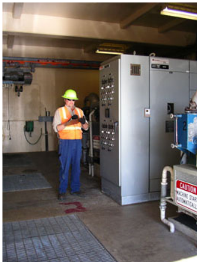
H Street Storm Drainage Station
