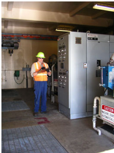
H Street Storm Drainage Station
