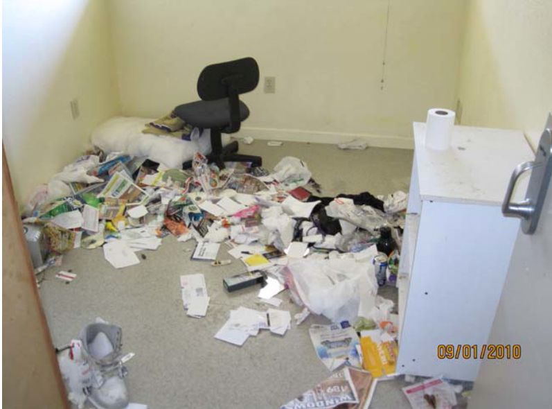
Vacant rooms “before,” with trash, abandoned items, broken locks, etc. –
