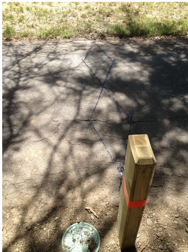
Figure 5: Pyroelectric Sensor (inside wooden post) and Inductive Loops (grooves in asphalt) installed in Sycamore Park.
