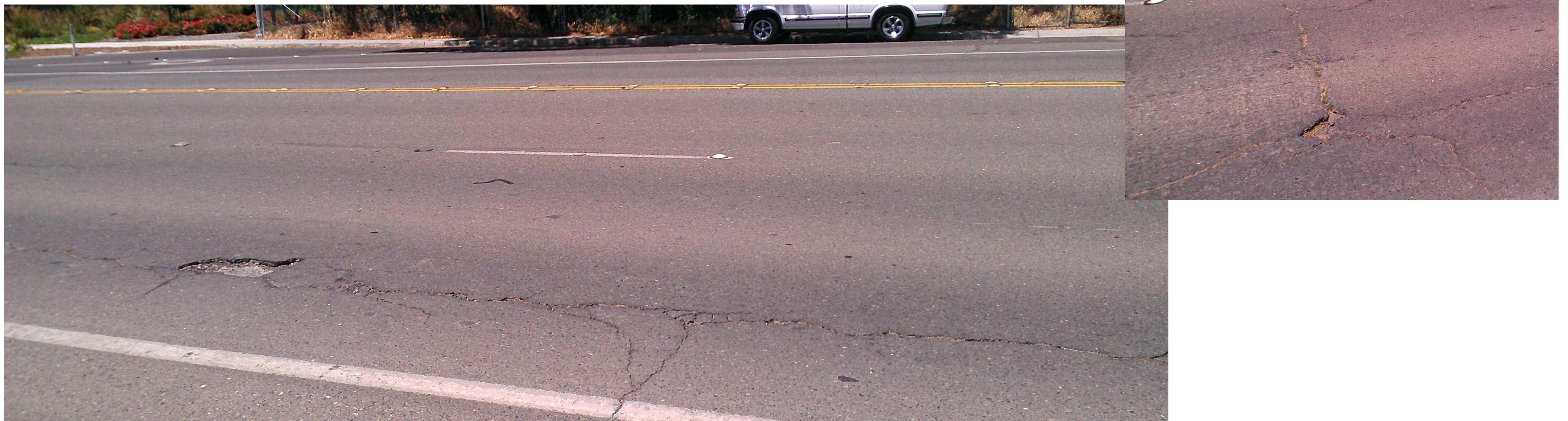
Potholes and cracking on Mace Blvd.
