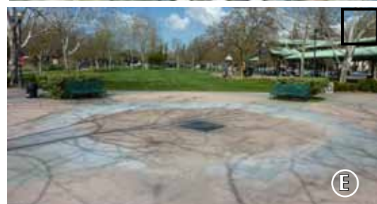
Fountain provides an iconic focal point and gathering space, but is not up to code and too steep to meet ADA accessibility requirements.
