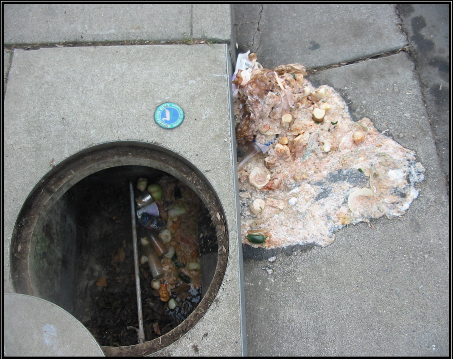
An Example of an Illicit Discharge in a Storm Drain that the City Cleared in Response to a Phone Call from a Concerned Citizen. Image shows City drain inlet # 19 on Eel Avenue.
