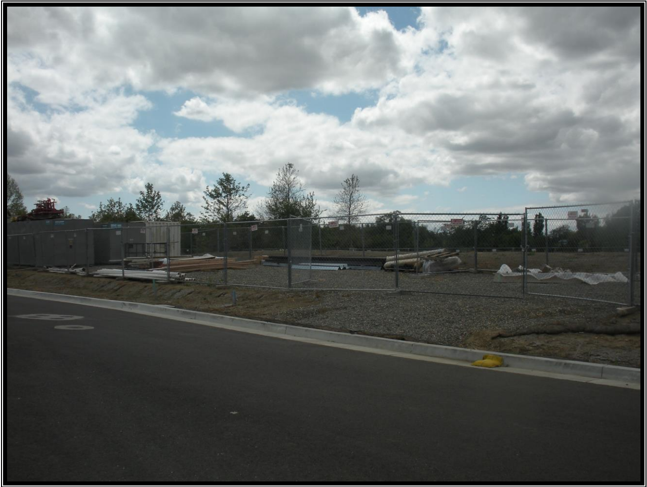
Sediment Control and Good Housekeeping BMPs at the Verona Subdivision (Second Street and Alhambra Drive).
