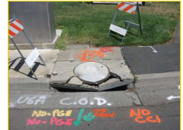
Revenue from the fee would be used to repair and replace damaged infrastructure.
