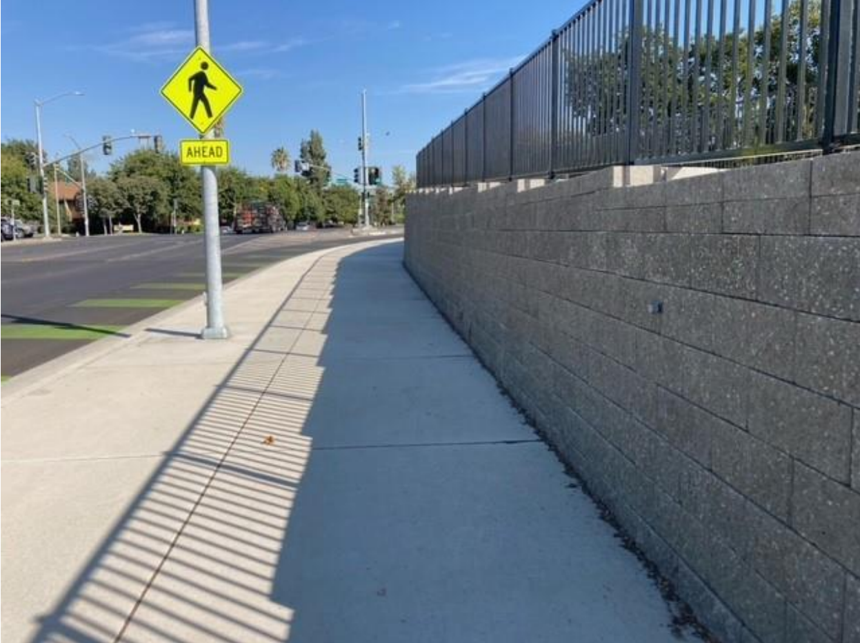
Facing North toward Covell on F Street, retaining wall increasing in height:
