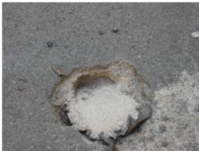
Figure 7 Formation of Clogging Crust on Filter Bed
