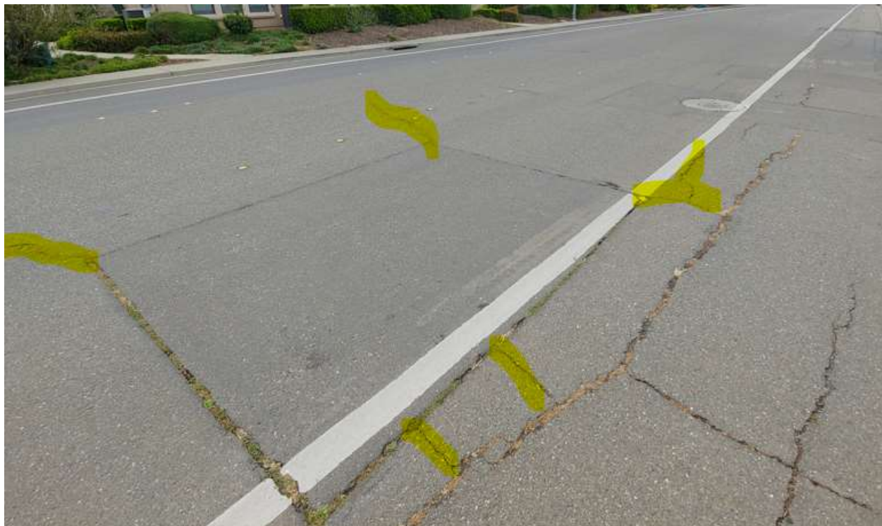
Figure 5. Propagating Cracks Near Patch on John Jones Road.
