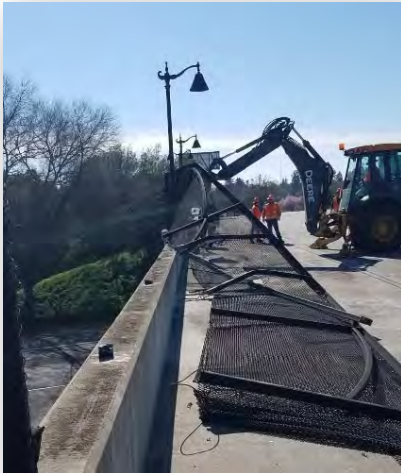
Damaged freeway screen on Mace Blvd.
