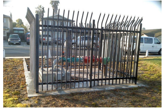
Figure 4-5. Typical park irrigation well
