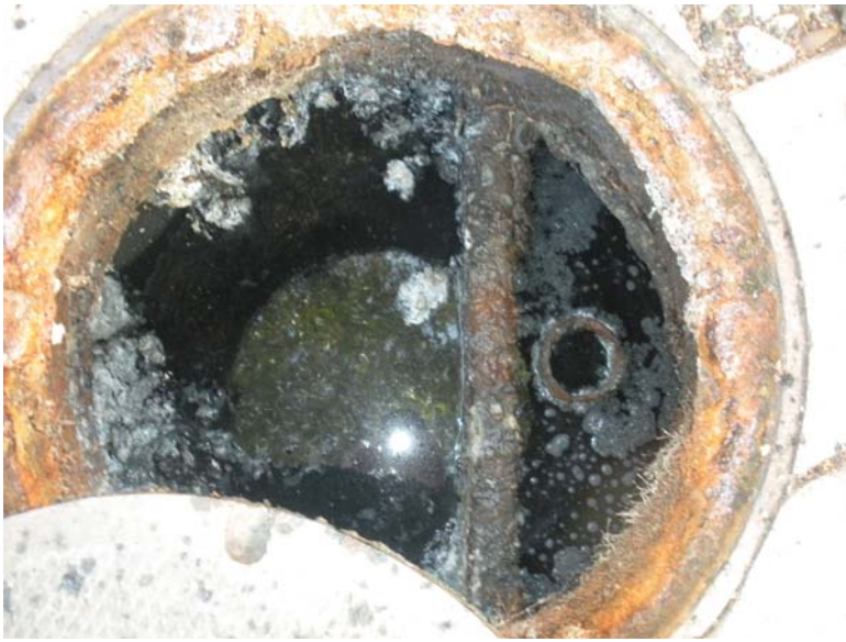
Unused in-ground interceptor located in the commercial complex. Has not changed since the last time I was there. Conditions appear to be anaerobic in the separator. 03/12/12
