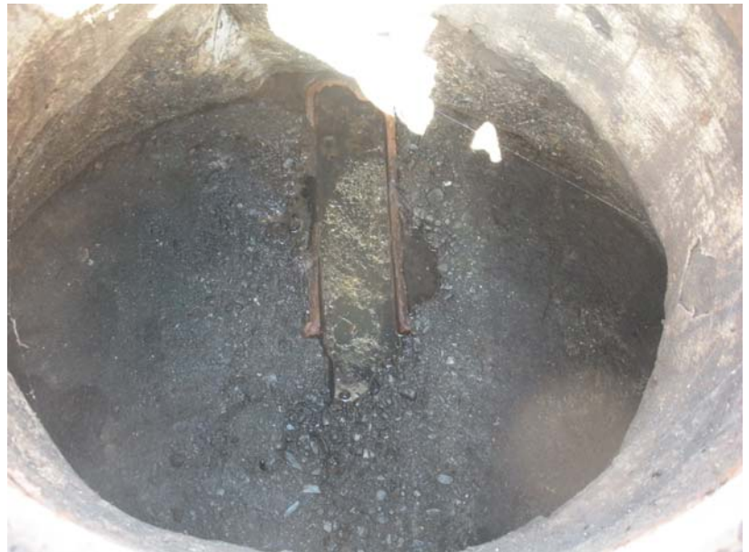
End of sewer line just up from where the SSO occurred. Standing water in the line 03/12/12.
