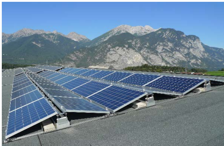
(Photo courtesy of Mounting Systems)
