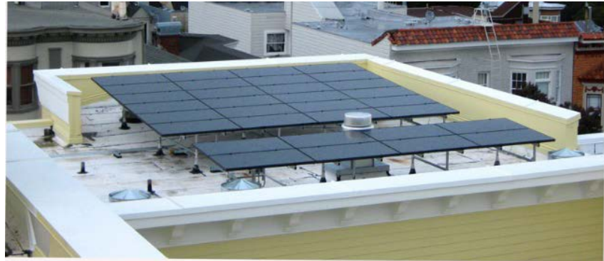
(Photo Courtesy of Sun Light & Power)
