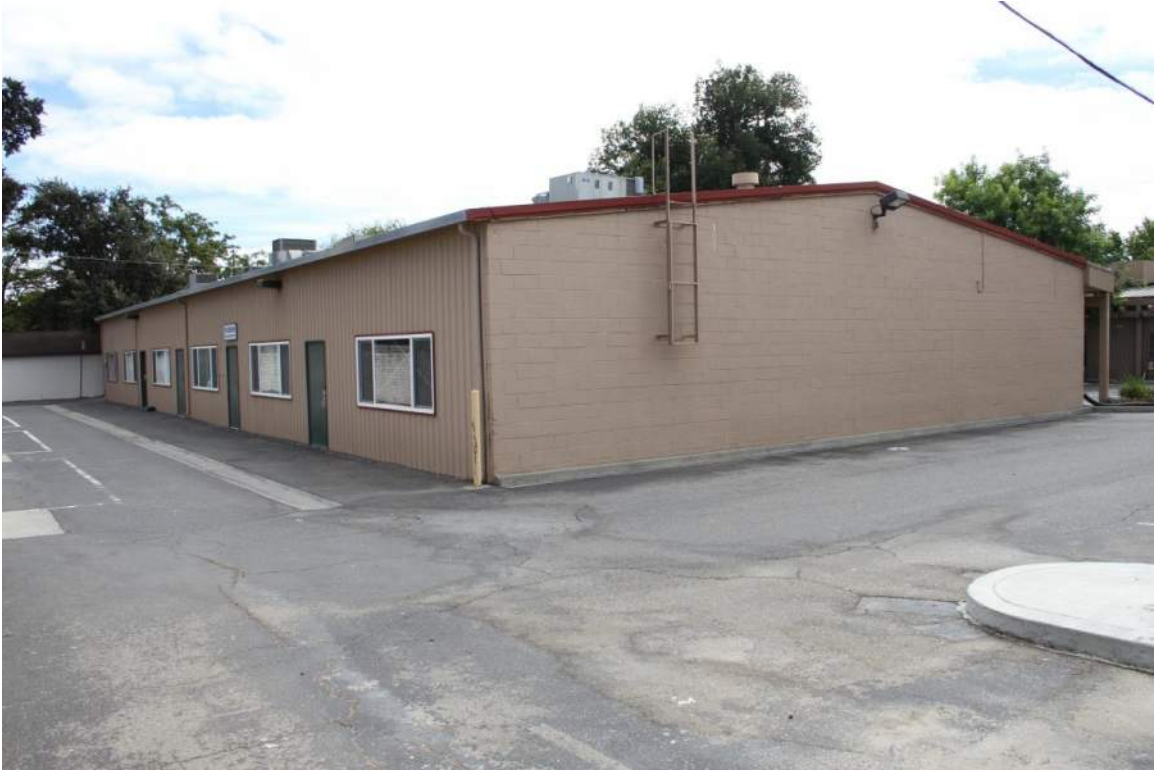
Photograph 11: View looking at the northeast elevation of the former motel. Note the exposed concrete block wall.
